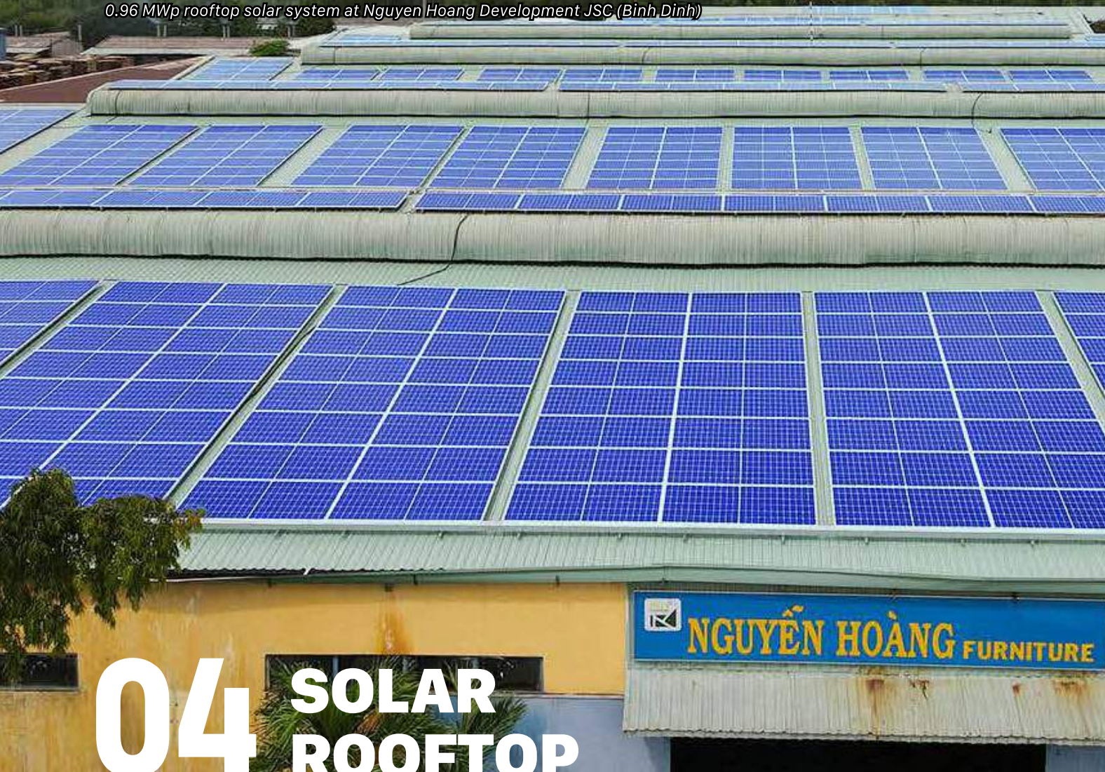
0.96 MWp rooftop solar system at Nguyen Hoang Development JSC (Binh Dinh)
